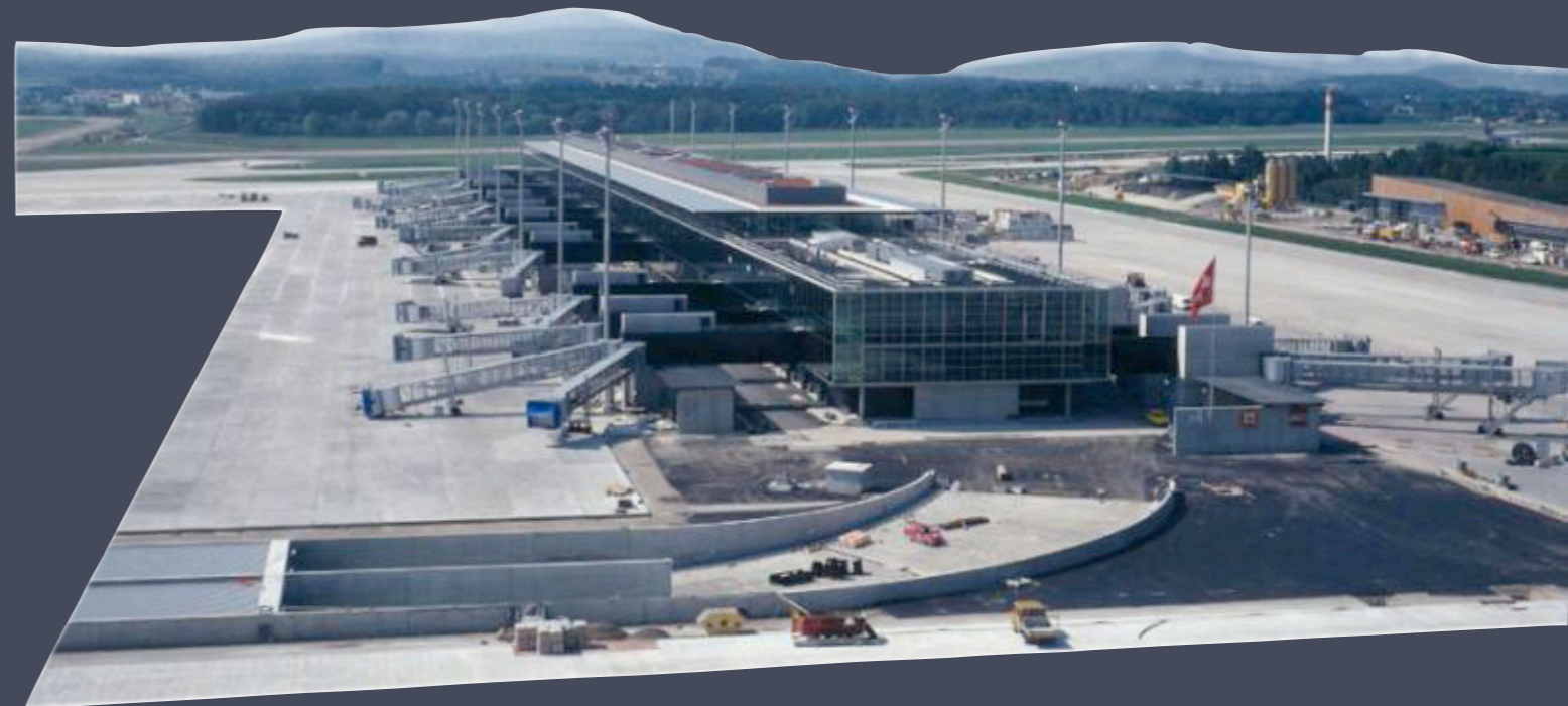
URBAN INFRASTRUCTURE International Terminal, Zurich Airport, Zurich
